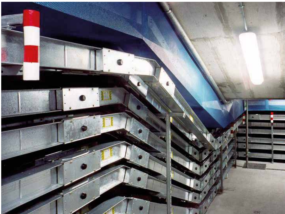
Example of high power distribution
